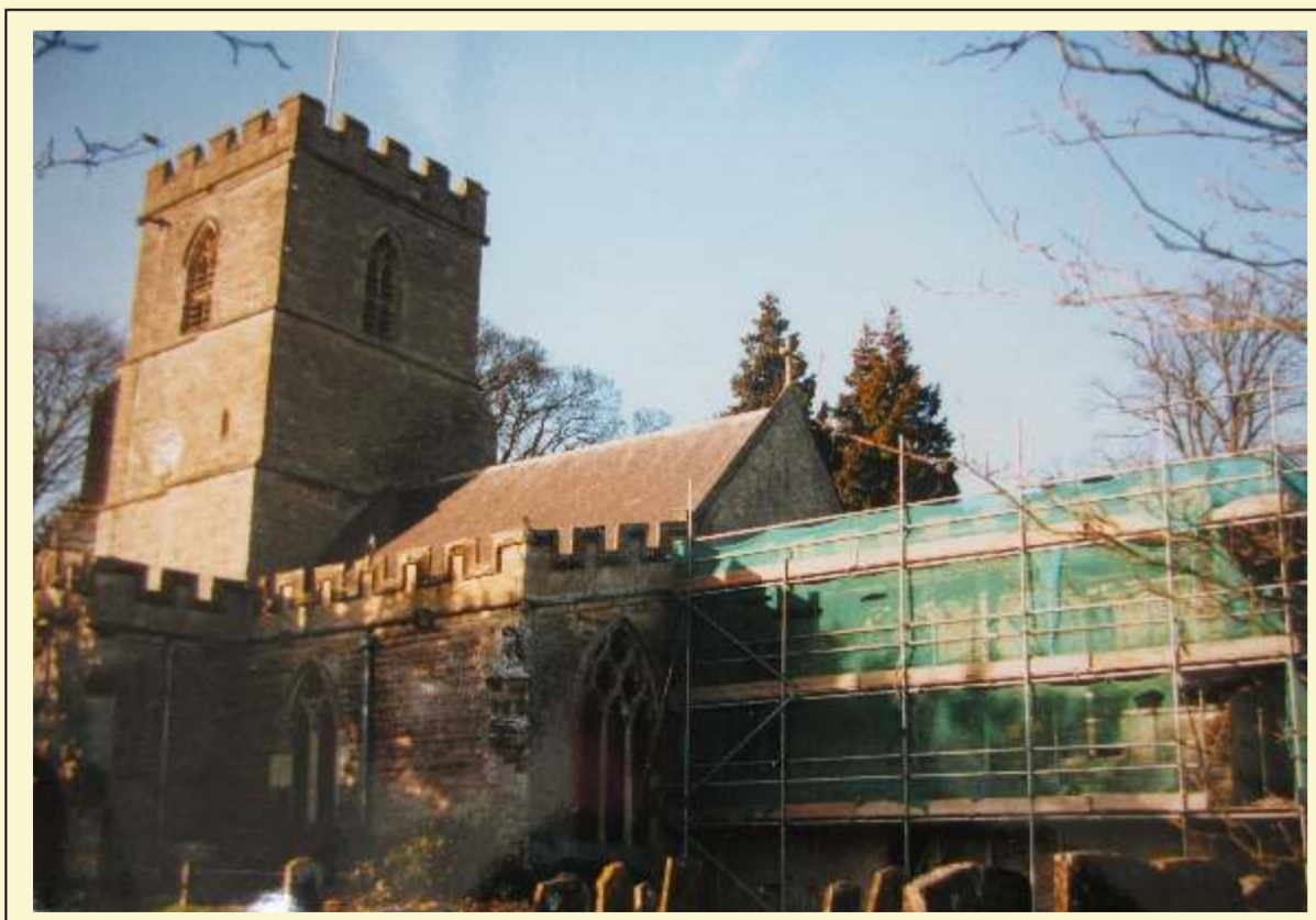
Autumn 1978. The church roof facing South was in trouble as the nail holes were expanding allowing the lead to shift. The Church Council together with their architect decided that it could be repaired with aluminium rather than lead. The Church roof appeal was launched and after some months of fund raising the roof was repaired in summer 1979.
